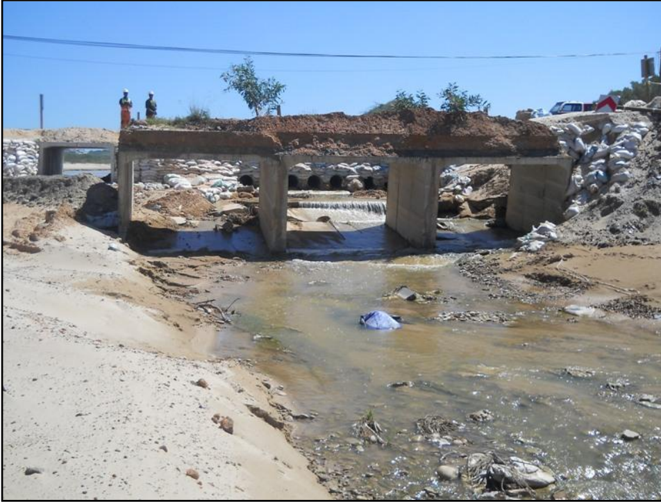
Figure 1: View of the crossing over the Sand River that washed away during the flood event in 2012.
