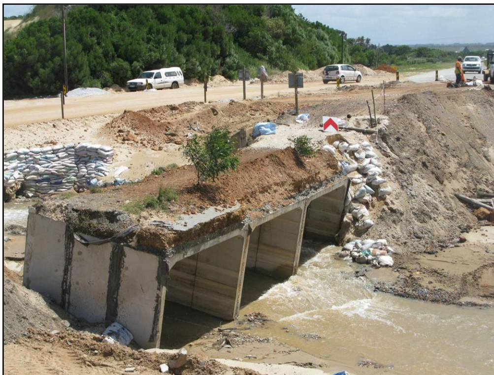
Figure 4: View of the undermined structure that requires replacement.
