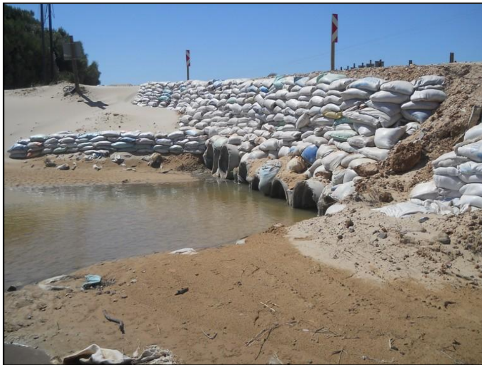
Figure 2: View of the temporary structure that is currently in place along the deviation allowing flow in the Sand River.
